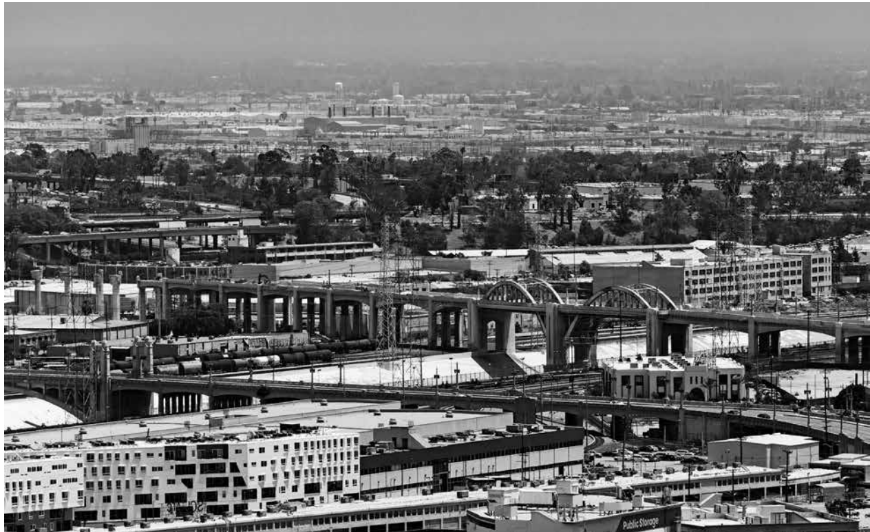
Demolition of Los Angeles' 6th Street Bridge over the Los Angeles River. Demolition was proceeding from the left (east) on May 27, 2016. The 1932 bridge with its two steel arches will be replaced by a bridge with a series of concrete arches..
