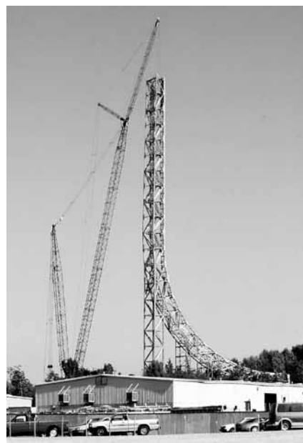
Construction of Magic Mountain's Superman Ride in May, 1996, required a crane nearly 500 feet tall
