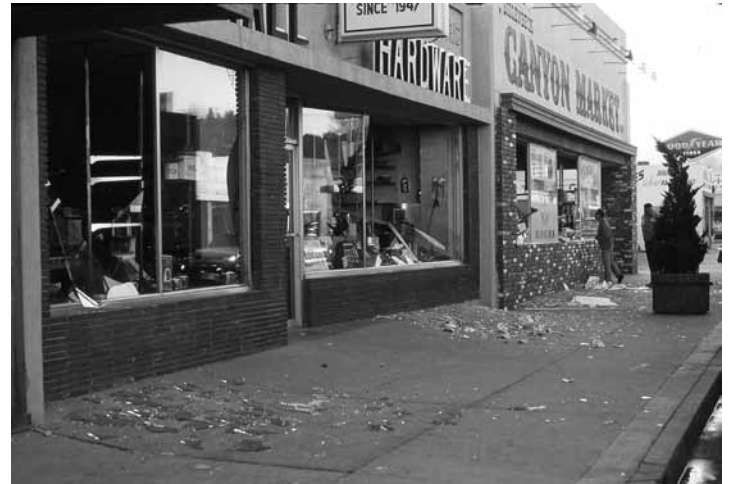
Most of the damage on San Fernando Road was broken glass
