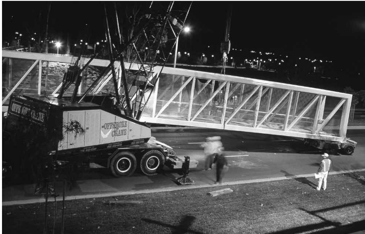
Bridge to Nowhere? The Paseo bridge over Valencia Blvd being lifted into place; December 3, 1993
