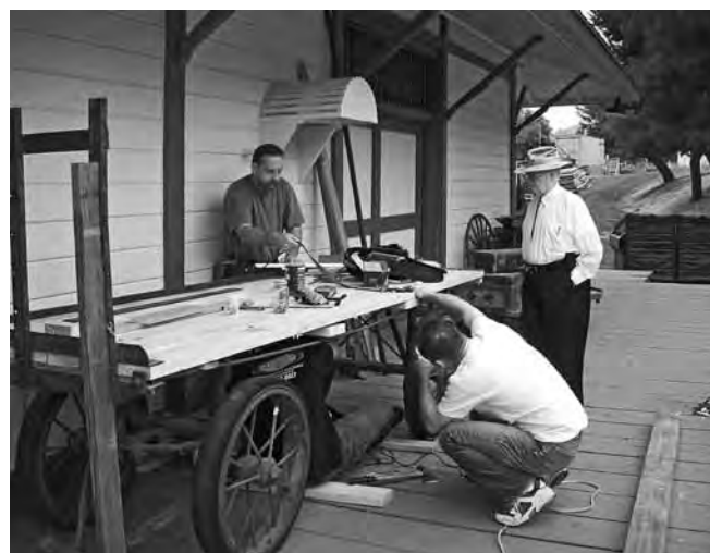
Community service volunteers, Ron, Jason and Mike replace deteriorating wood on the Railway Express wagon on the dock at the Station as John Lesperance “supervises.” Soon, it will again sport its bright red and green colors. Thanks also to Tom Burgh and the Santa Susannah crew for a steel ring to use for the tongue.
